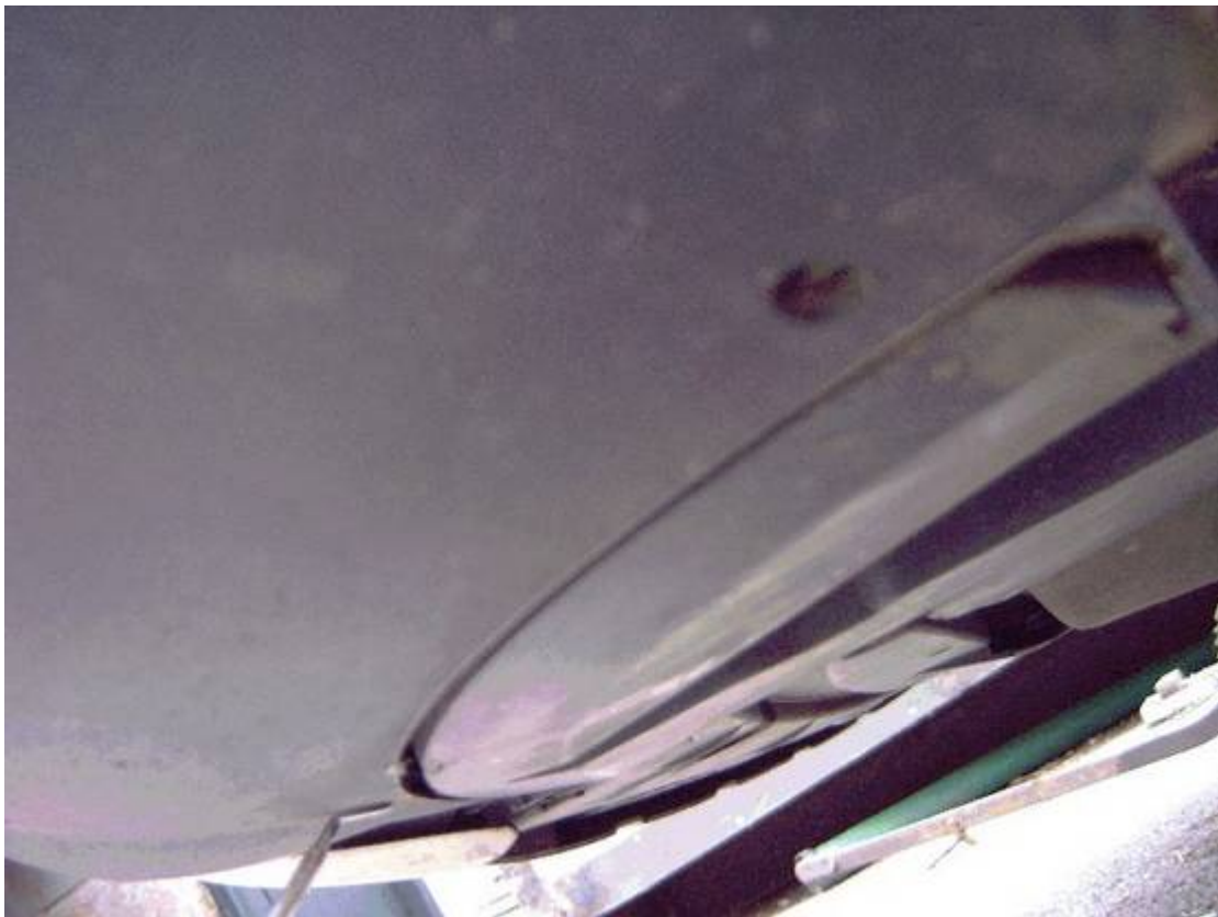
Push dot fixings on lower edge (1 missing)
